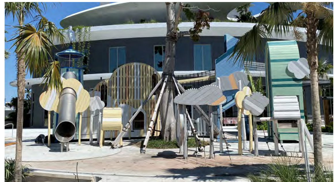
The under-construction playground at Waterfront Park, west of Bal Harbour Shops on Bal Bay Drive. Play components include multiple climbing towers (3-4), slides, and bridges.
